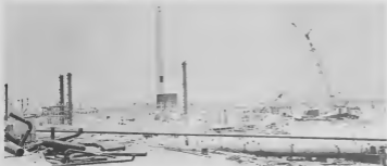
The first towers and the furnace for the Vacuum Pipestill are set in place. E promer towernan y lorno pe e Vacuum Pipestill ta ser poni na nan luger.
